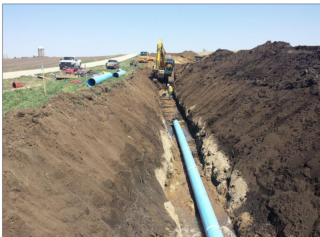
The first section of 24-inch steel pipe is installed between Luverne and Iowa border last month.
