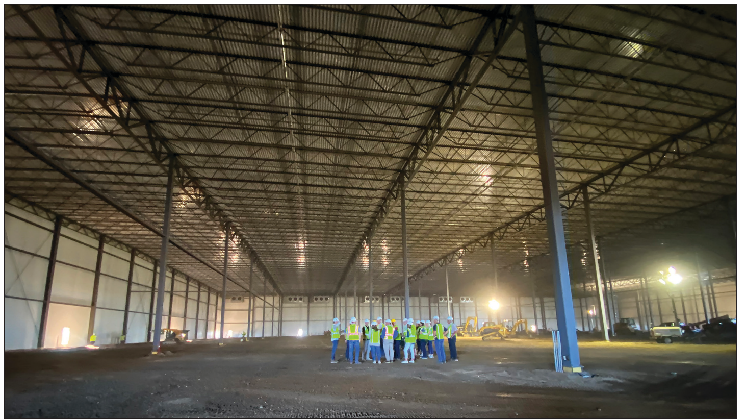
The Luverne City Council and Rock County Commissioners toured the Lineage freezer storage warehouse Aug. 30 being constructed in the Luverne Industrial Park. The gigantic building is roughly 400 feet by 450 feet with a 48-foot ceiling.
