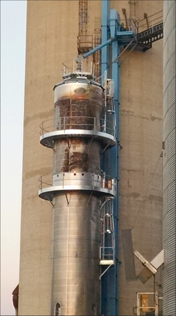
Mavis Fodness photo/1008 Fire CHS Magnolia A closer view of the dryer reveals significant damage to the structure at the CHS Magnolia elevator.
