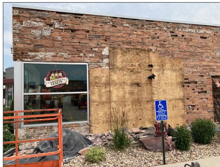
The expansion project will also address deteriorating bricks on the west wall of the History Center.
