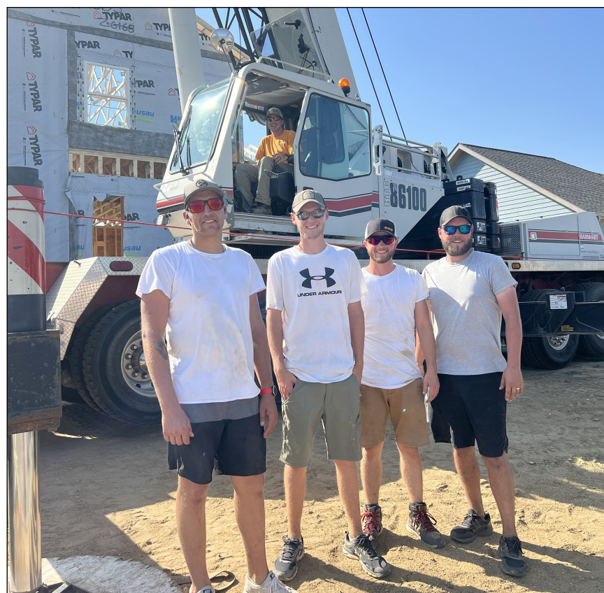
Five Luverne High School graduates (from left) Dalton Jacobsma, Joe Guy, Matthew Sterrett, Jake Guy and Brian Barnhart (in crane) came together last week to set the framing and trusses for a home being built for Angela and TJ Newgard (a Luverne teacher). Submitted photo
