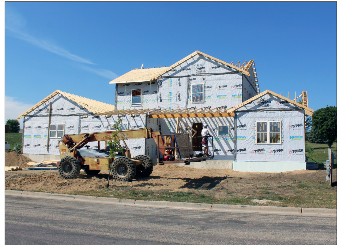
On Monday, Aug. 28, Jake Guy (driving the telehandler) and Matthew Sterrett (on scaffolding), along with Joe Guy (inside), complete roofing work at the home they are building on Manfred Drive. The three are all Luverne High School graduates. (Submitted photo)
