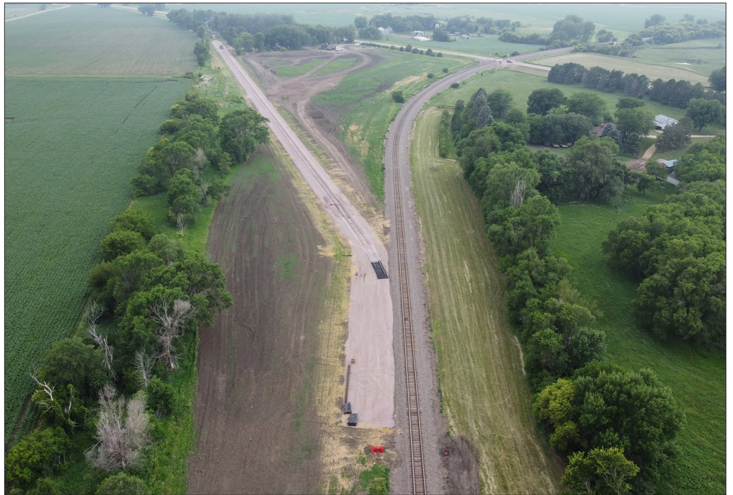
This drone photo shows where a switching system is ready for installation near Manley. This portion of the Buffalo Ridge Railroad rehabilitation project has been delayed for the past 14 months by the officials at the Burlington Northern Santa Fe Railroad. Work on installing the switching system is expected to begin in September. Pictured below, More than 10,000 railroad ties are expected to be replaced on the Buffalo Ridge Railroad as part of a $33.9 million rehabilitation project for the rail line that runs through the southern half of Rock County and ends in Worthington in Nobles County.
