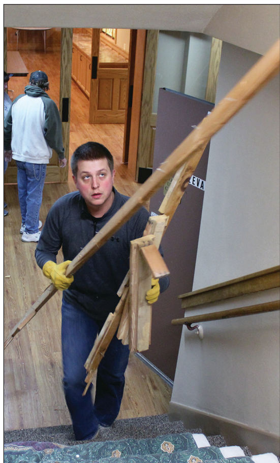
Caleb Ellingson carries construction debris from the demolition of the Bethlehem Lutheran Church kitchen Saturday morning.
