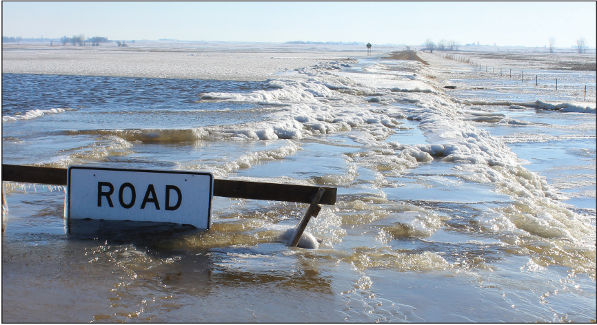
Mavis Fodness photo/0321 Flooding March 15 A "Road" sign (intended to be a "Road Closed" sign) is all that is visible Friday morning along 161 st Street two miles south of Kenneth. The township gravel road was taken over by melting snow Thursday and by Friday morning was covered by frozen slush and water.
