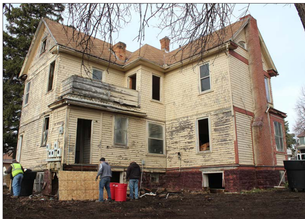
Lori Sorenson photo/1208 condemned house
