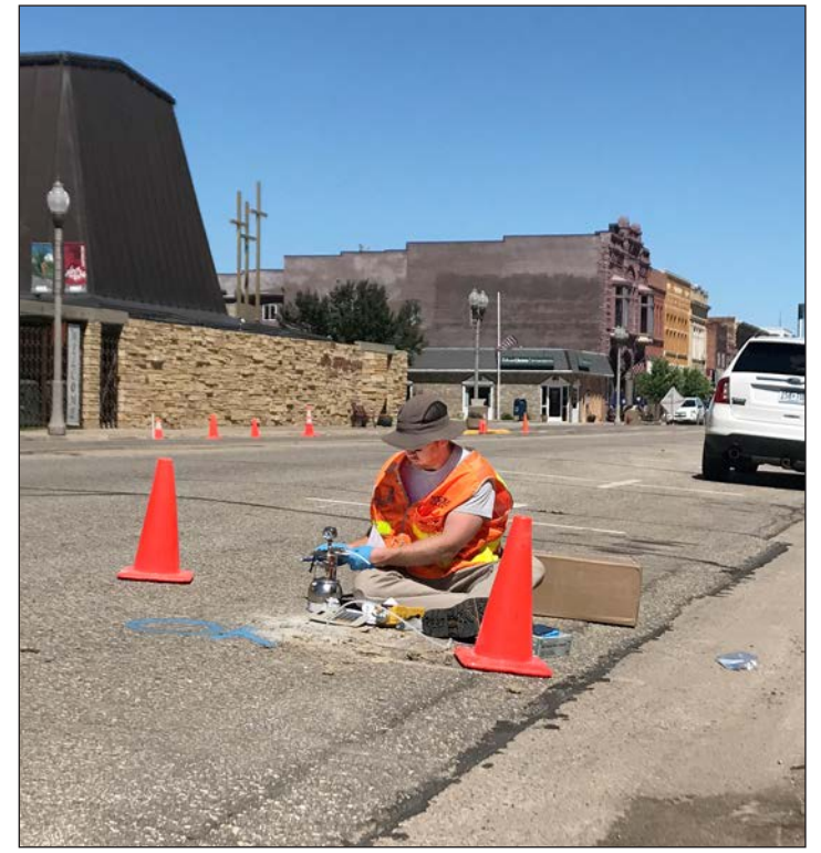
Lori Sorenson photo/0622 petroleum leak
