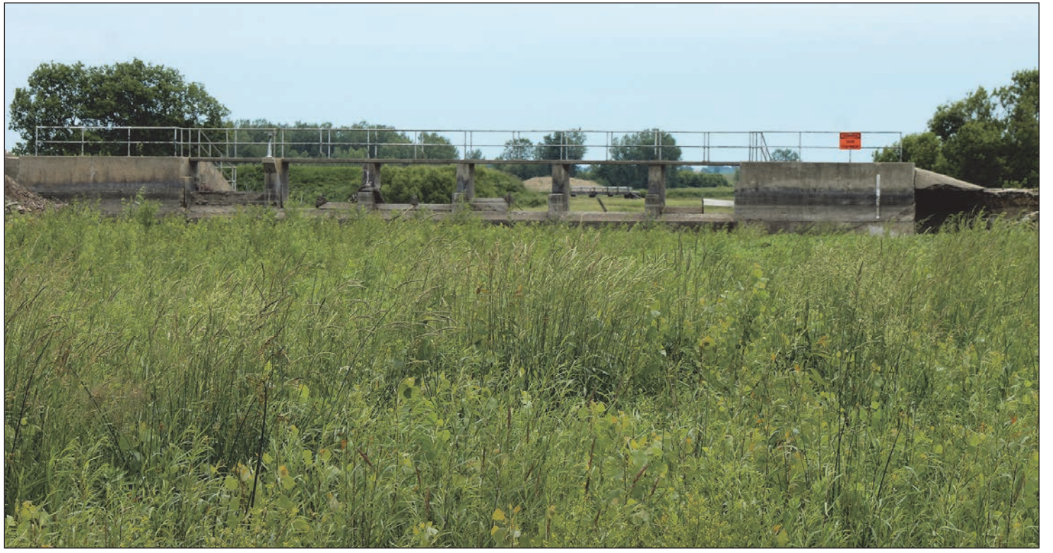
Mavis Fodness photo/0618 Flood After June 2014, flooding removed a portion of the dam at the Blue Mounds State Park (above). The Lower Mound Lake at the park has been reduced to a grass marsh.
