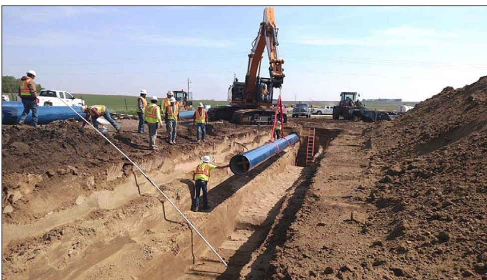
This photograph shows the first section of 24-inch steel pipe being installed.
