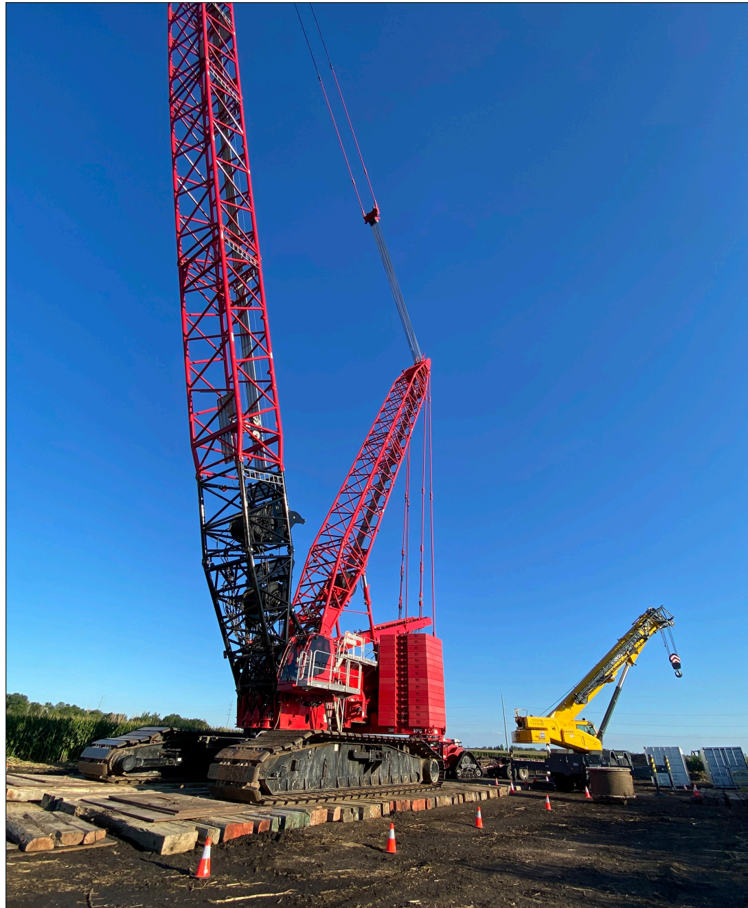
The main erection cranes weigh 716 tons and need to rest on “crane mats” comprised of wooden planks 5 feet wide by 20 feet long by 1 foot thick to displace their weight on the ground. Smaller cranes with 300-ton lifting capacity are used to assemble the lower tower sections and build the rotors on the ground before they’re lifted in place. (Lori Sorenson photo)
