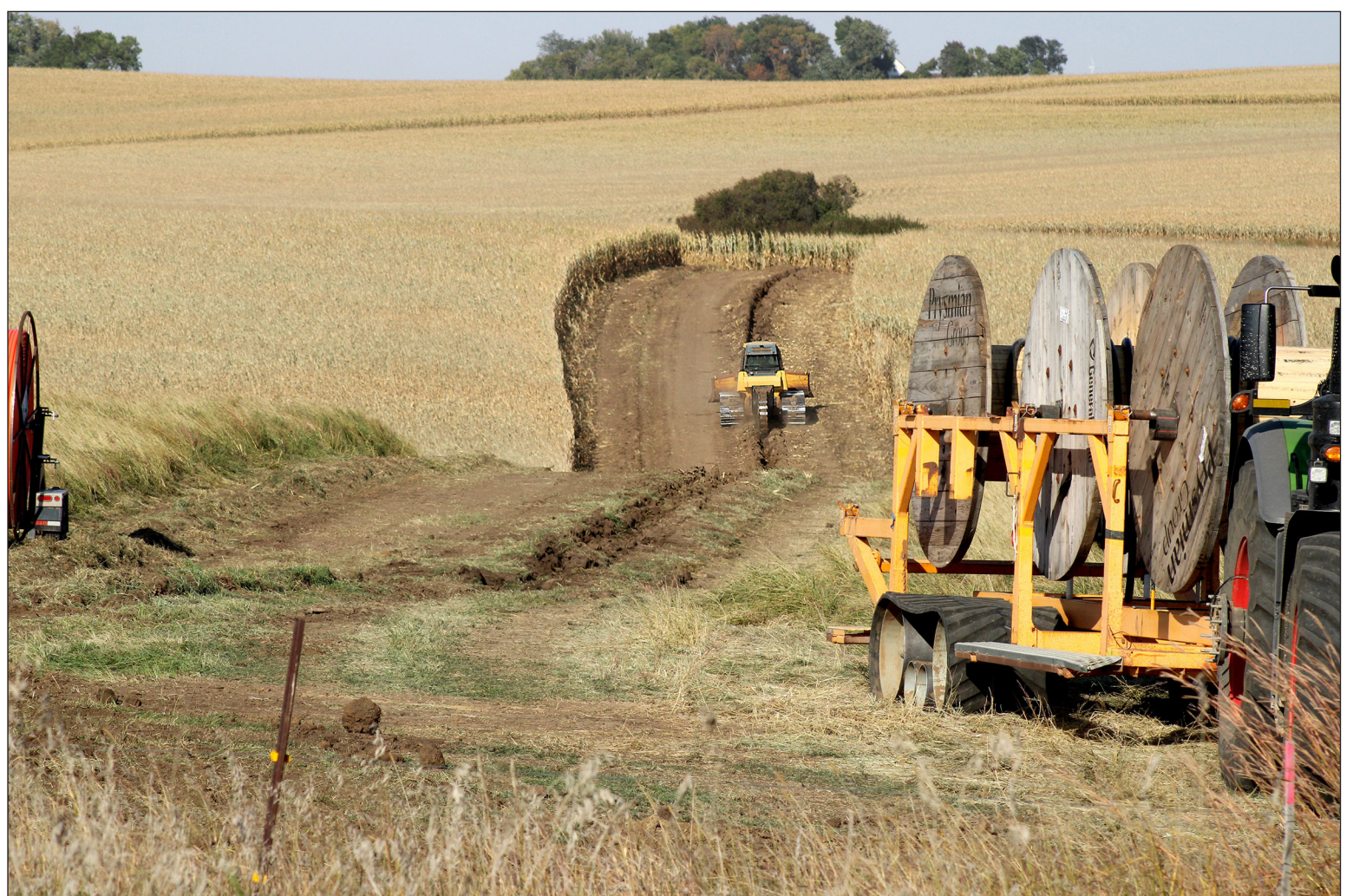
Each turbine requires underground "collector" cables to deliver electricity to the grid. These 200,000 feet of cable are trenched in about 4 feet below ground level, and the trenching paths are roughly 90 feet wide, in order to accommodate equipment. This means widespread crop loss and damage to field tiles. All losses and damages are compensated by NextEra. (Lori Sorenson photo)
