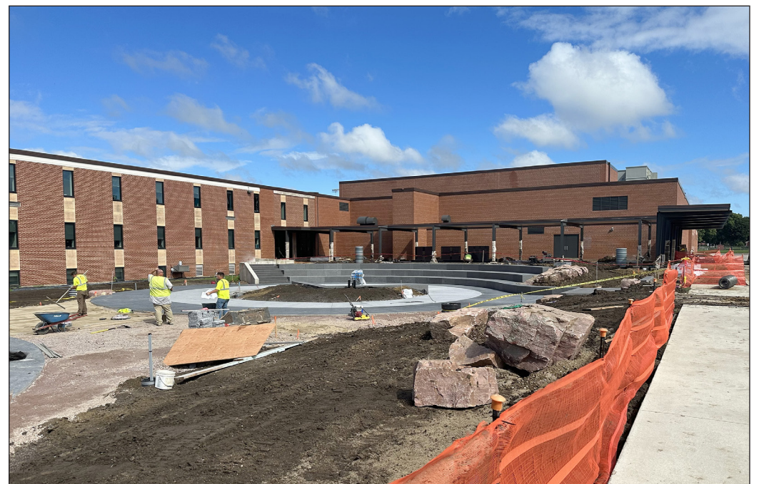
Layers of granite and concrete begin to take shape at the Alumni Garden construction site Monday morning. Dedication is planned for Oct. 6 during homecoming week.
