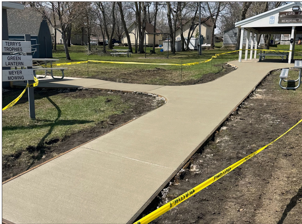
A new sidewalk was poured in the Hardwick city park last week as part of an age-friendly grant through the Minnesota River Area Agency on Aging. It's part of several projects the $10,000 grant will add to the park before an unveiling celebration occurs in late June.
