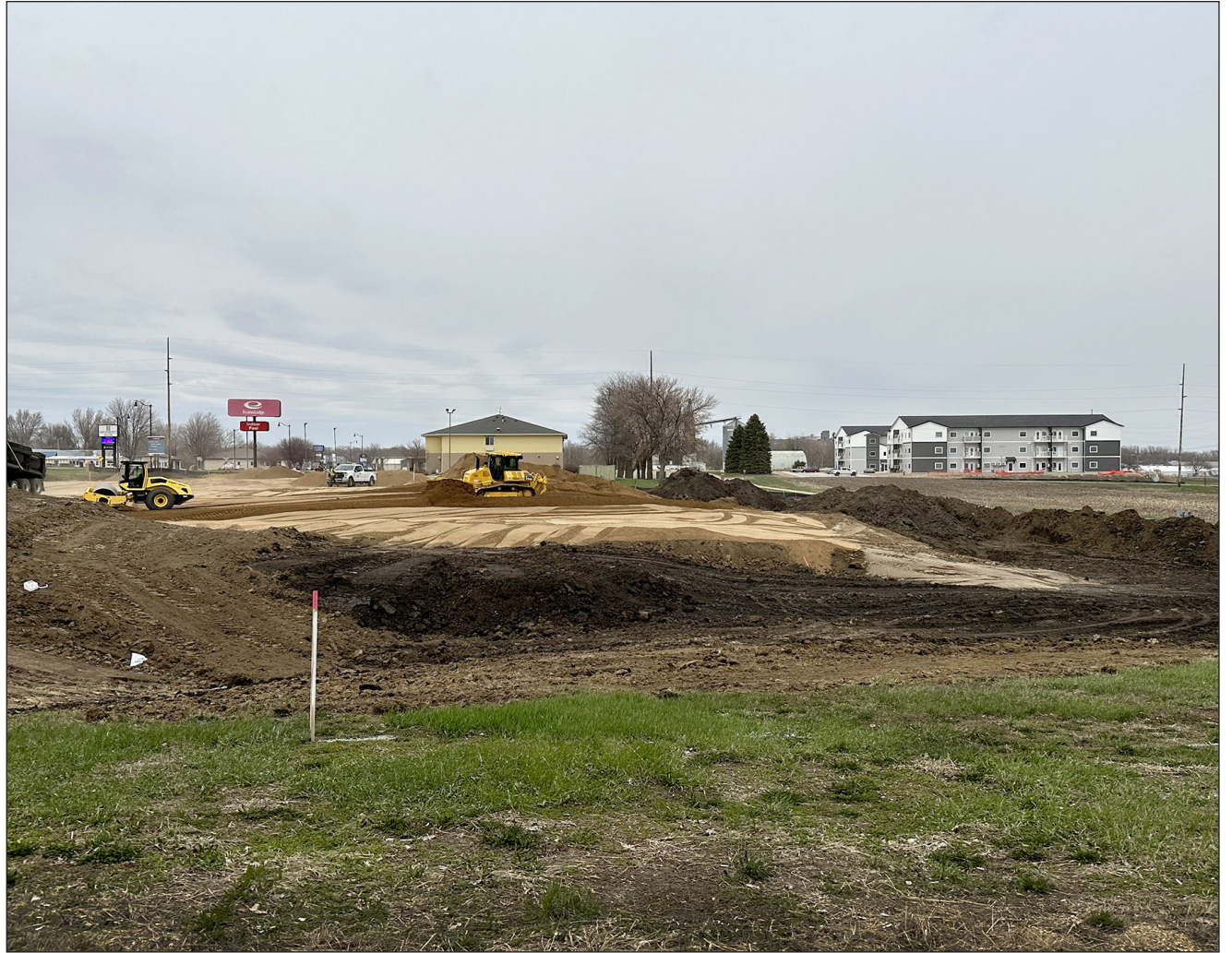
Earth moving equipment is on site to bring a Kwik Trip to South Highway 75 in Luverne.
